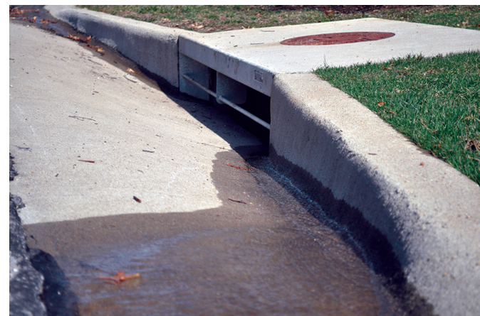
Water that flows into stormdrains is not treated. It drains directly into county streams.
